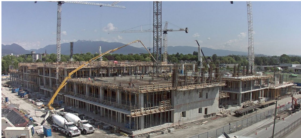
The concrete floors for levels 1 and 2 of the new St. Paul's Hospital are now complete with teams working on levels 3 and 4. By the end of the year, the hospital should be up to floor 7. (Photo taken May 25, 2023)
